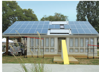
Roof-integrated PV system
